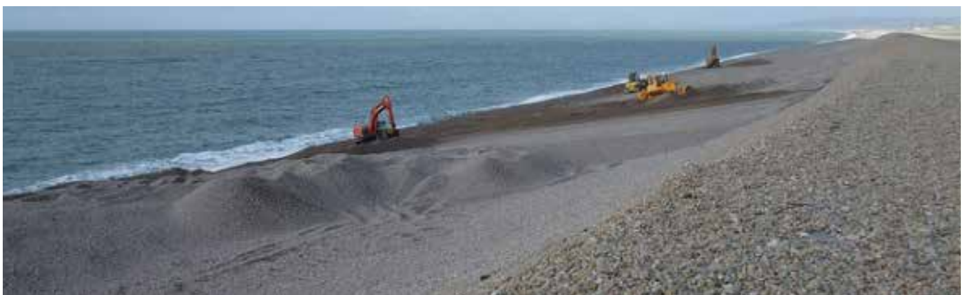
Figure 3.18. Replenishment and reprofiling on the shingle at Chesil beach, Dorset: This work was undertaken in order to increase protection to the community of Chiswell following significant storms (© Environment Agency).
