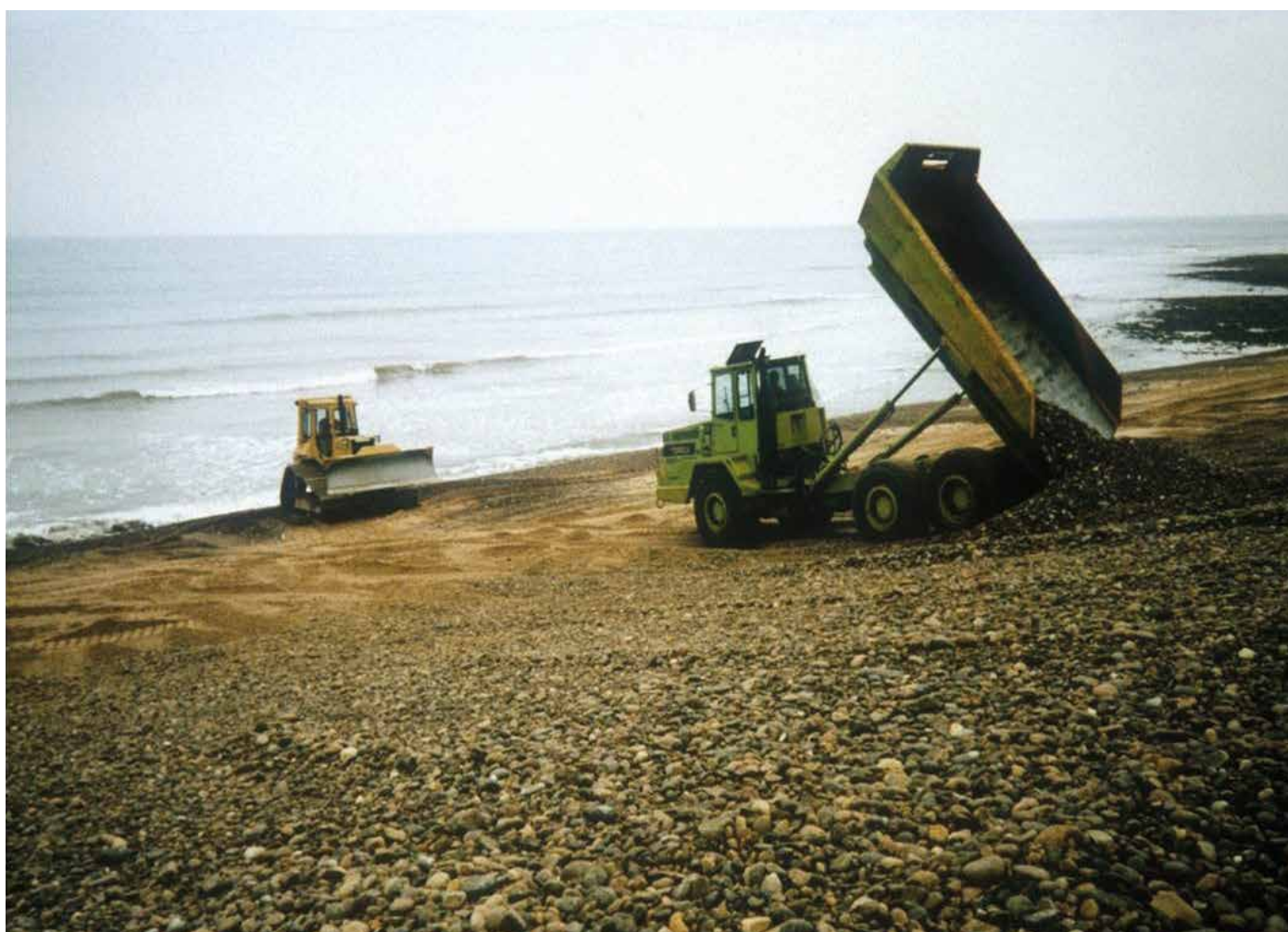
Figure 3.19. Shingle restoration at Spey Bay, Moray – Scotland's largest shingle beach (© Sally Gemell).
